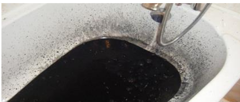
FIGURE 4: There is a foul waste-water smell and in some cases waste reflux into sinks and baths (as shown here)
