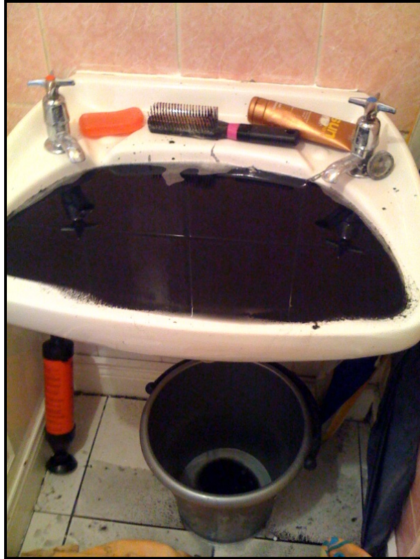
Plate 2-2 Wastewater Backup Observed on June 28 th 2010
